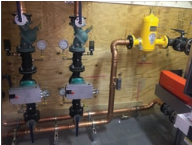
Flow is provided by two Wilo ECM pumps.
