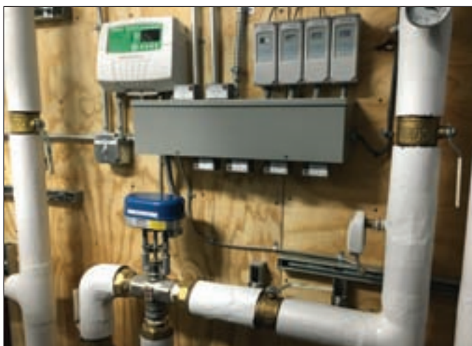
Supply water temperature is maintained at a steady 120 F by the electronic temperature control and the stainless steel motorized tempering valve.
