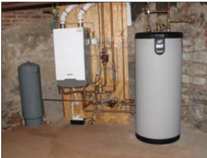
Photo 3: The replacement system consisted of a Triangle Tube Prestige condensing natural gas boiler. We also replaced an electric water heater with a Smart 80 stainless steel indirect fired DHW tank.
