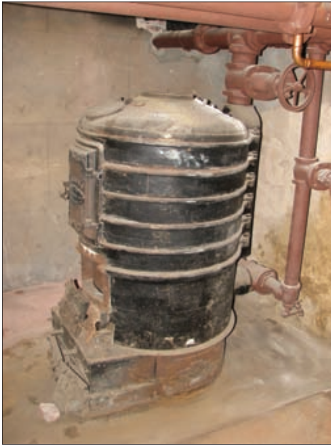
Photo 2: The original Gurney coal-fired boiler was still in place but valved off.
