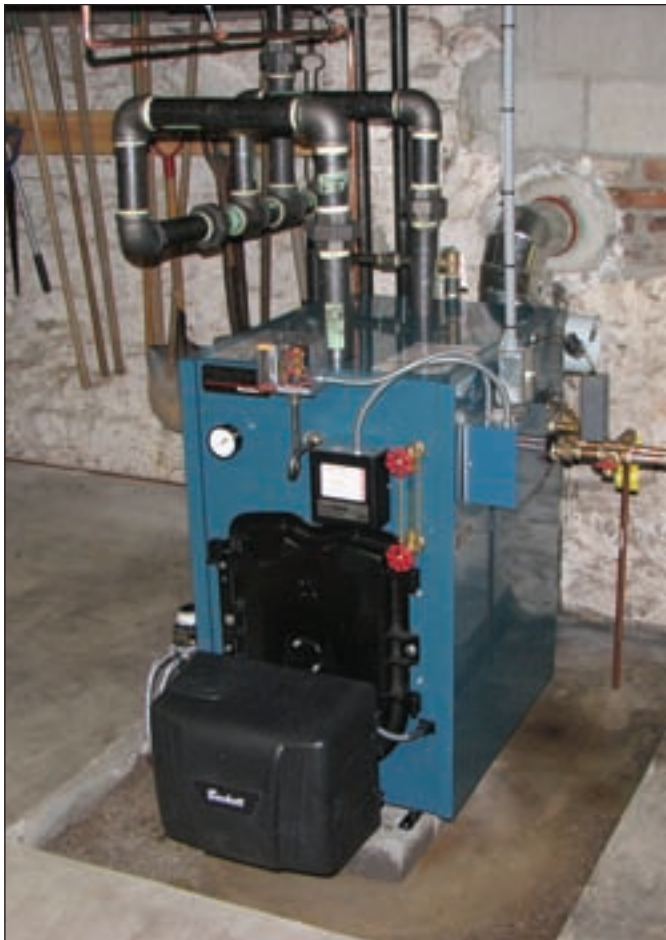
Photo 7: We replaced the second boiler more recently employing a Burnham MegaSteam cast iron oil boiler.
