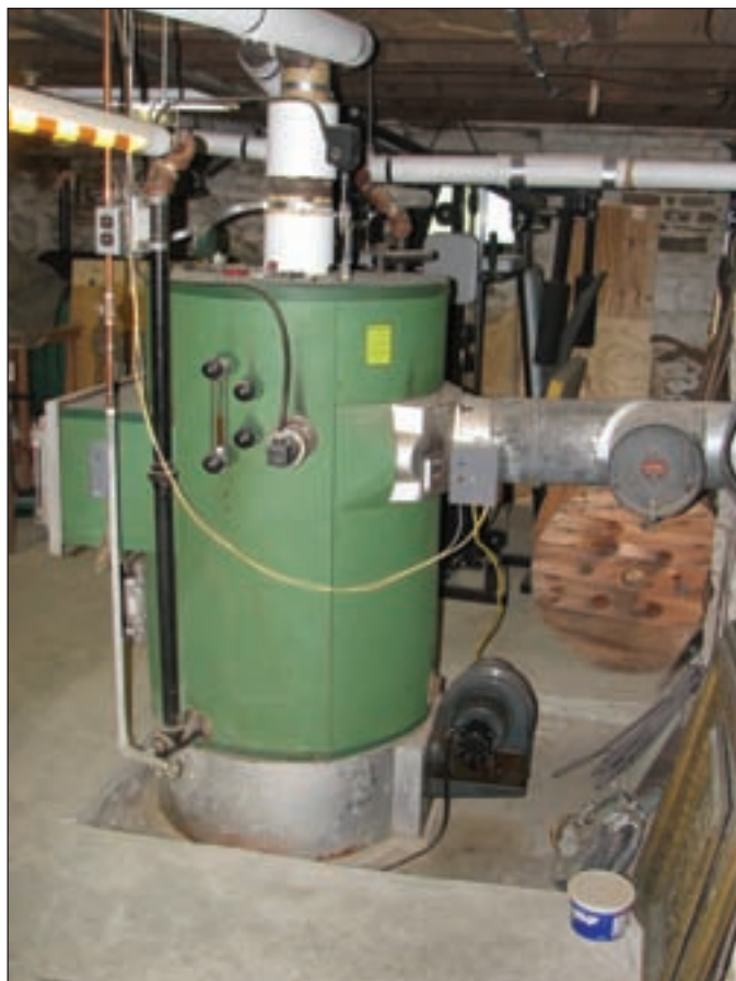
Photo 5: The current owner's grandfather was a steamfitter and installed two steam systems in the 1940s. He installed two Kewanee steel oil-fired boilers connected to one-pipe steam systems.
