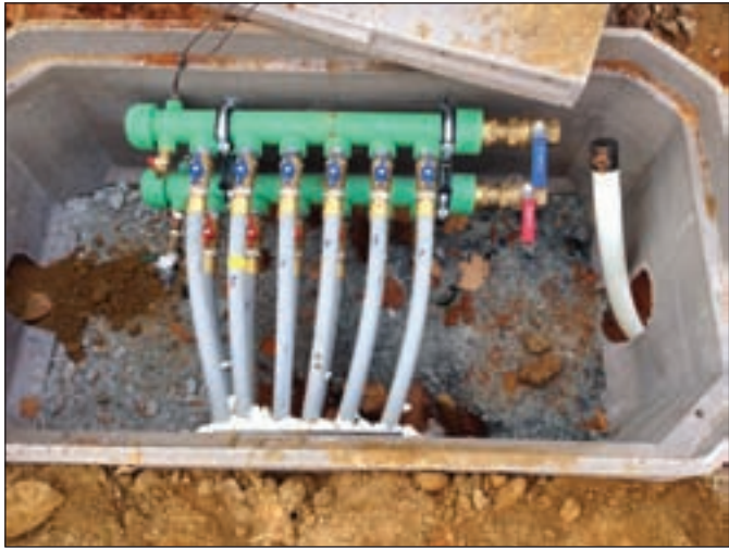
A Legend Hydronics geothermal manifold installed in a Foley Mechanical jobsite in Bethesda, Md.
