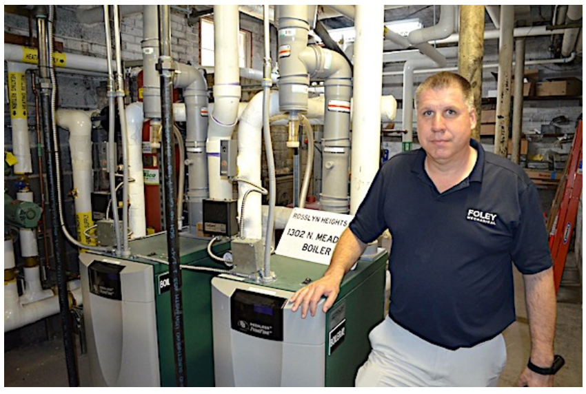
Dan Foley stands beside two Peerless PureFire boilers. The heating system consumed 47,017 cubic feet of gas before the retrofit and 28,729 cubic feet of gas after the upgrade for a total savings of 40%.
