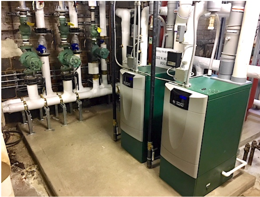
The boiler room includes two Peerless PureFire condensing gas boilers, which provide heat and domestic hot water (DHW) to the building.
