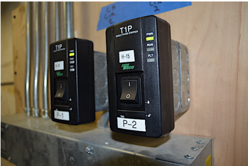
All line voltage wiring and switches, which serve the boiler system, were upgraded.
